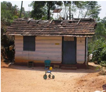
Fig. 2 A house damaged by lightning
