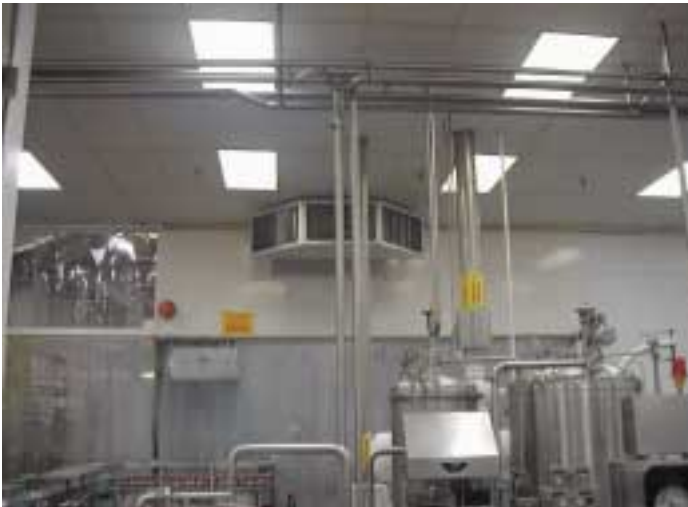
The carbon dioxide exhaust fans in the filler room are capable of 15 air changes per hour at Springs Inc., which is a major soft drink manufacturer and a large local Coca-Cola franchise distributor located in Huntsville, Alabama.
