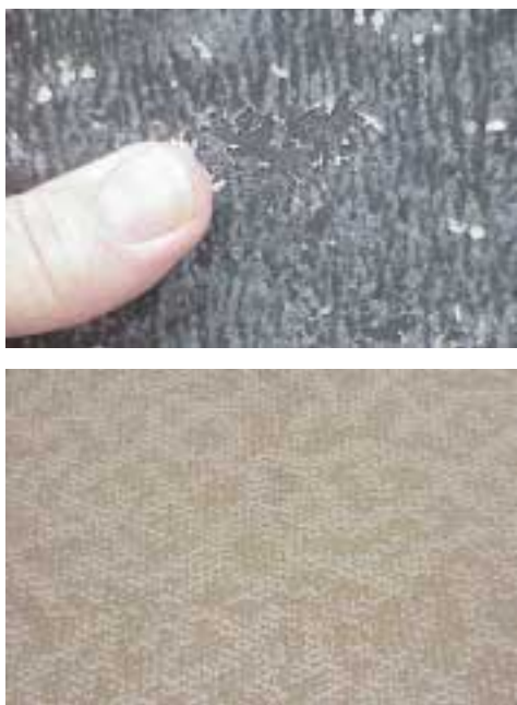
Figure 4. Carpet tile was curling and debonding on the slab-on-ground.
