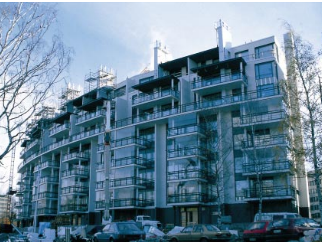
The 'Merikannonranta' is a construction research site in Helsinki where structural humidity measurements were studied at a built-in-site seven story residential building. Vaisala's HM44 moisture probes were used to monitor the moisture content of the structures throughout the construction process.
